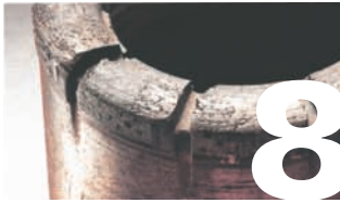
LOSS OF INSIDE DIAMETER
