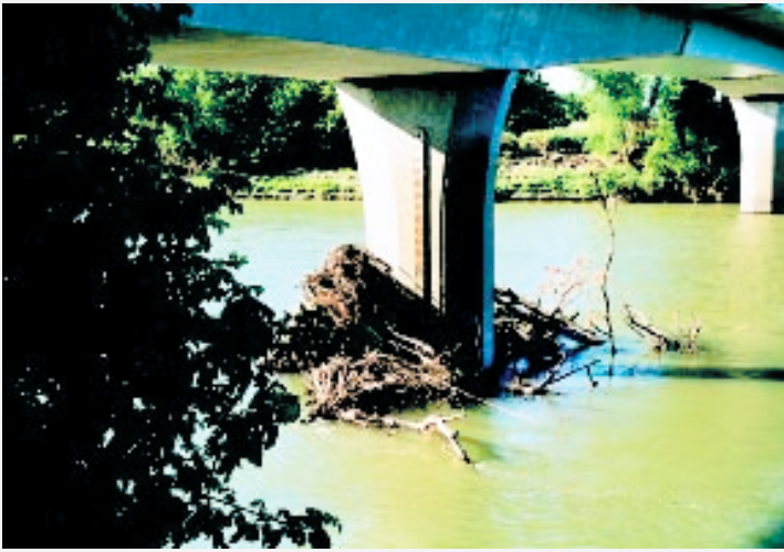
River with debris
